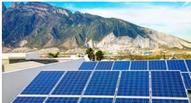
Rooftop solar PV, pxhere.com
